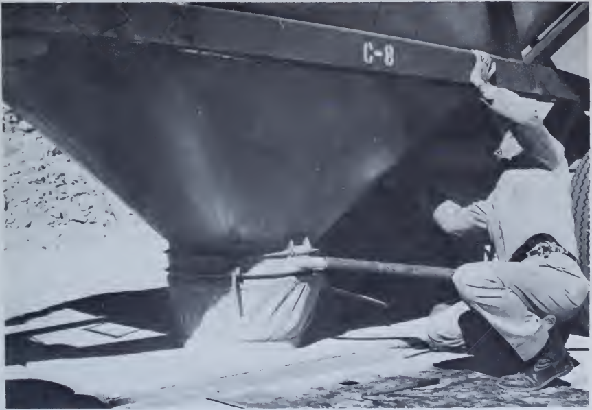
Figure 90.—Connection used in dumping cement from transport trucks to receiving hoppers of cement storage silos at Glen Canyon Dam, in Arizona. This arrangement minimized cement loss. P557-420-04599.
